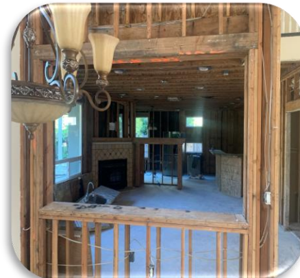
Pray for Our House Repairs
